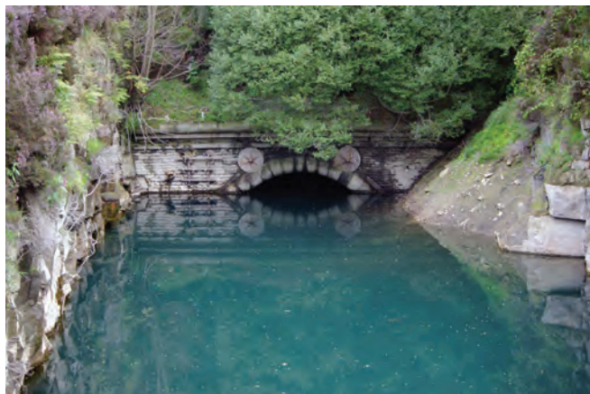
The flooded south portal of Queensbury tunnel in 2010. The water level was low that year; the portal was usually completely under water.
